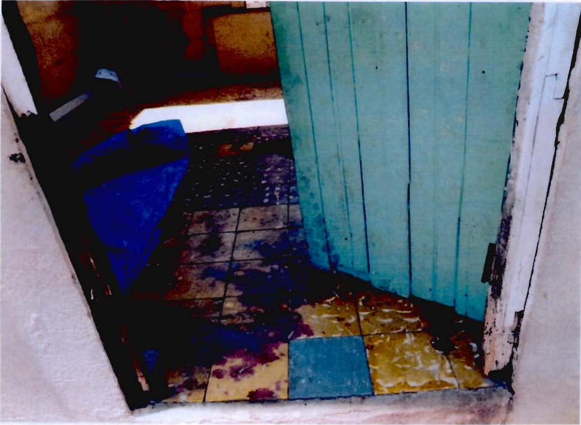
Figure 1: The damaged entrance to the house
