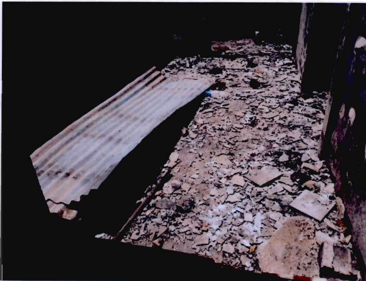
Figure 2: The living room area of the house which was completely gutted by fire
